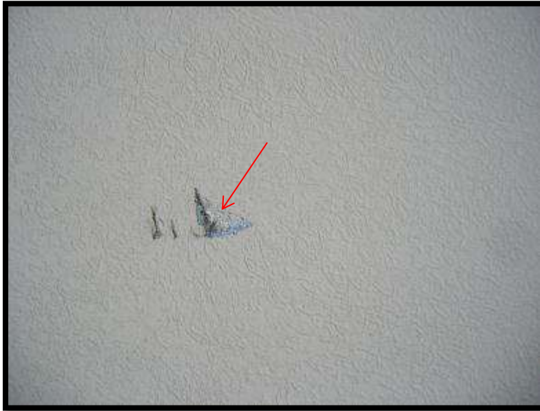
Photo 21: Gouge on EIFS wall (North elevation).
