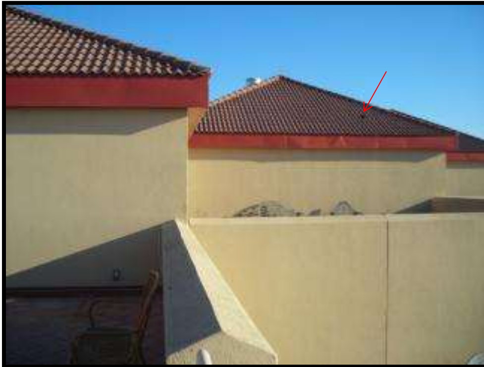
Photo 6: Missing/dislodged roof tile along upper roof (View from balcony of Unit 704).
