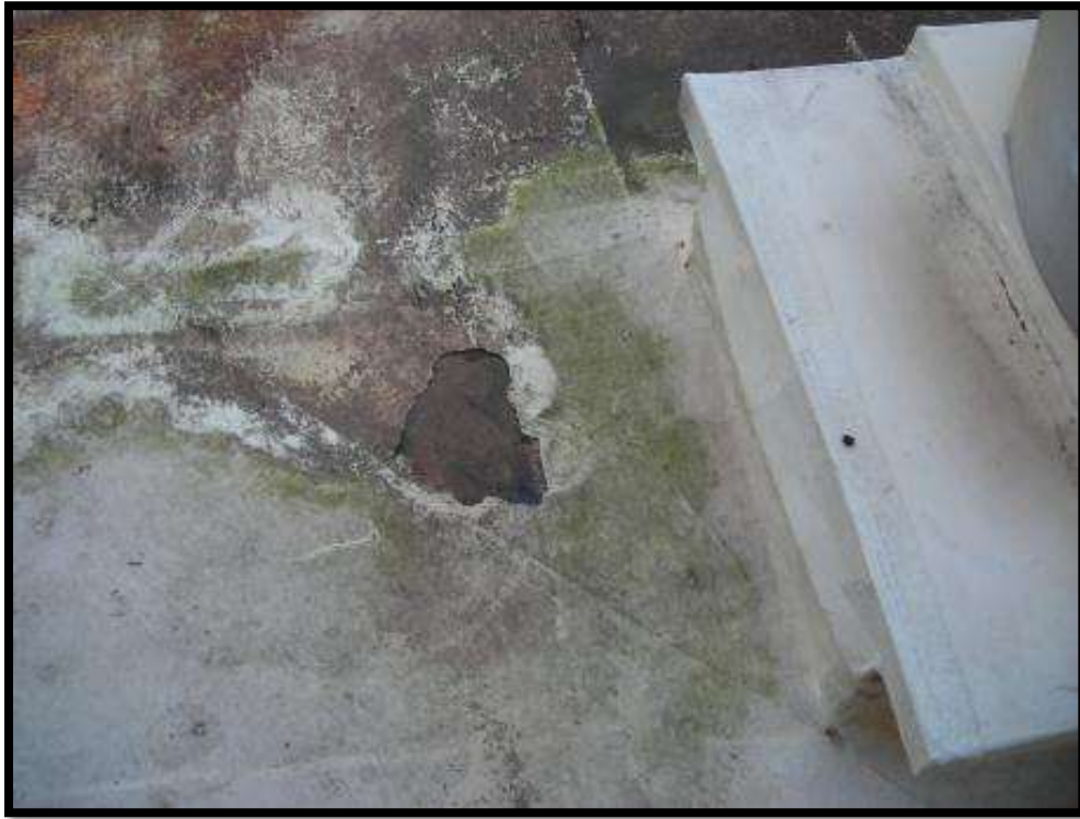
Photo 9: View of aged and deteriorated roof membrane (TPO).
