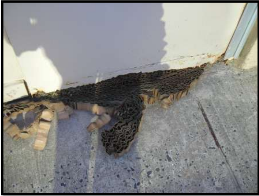
Photo 23: Damage to metal door sill (North elevation).
