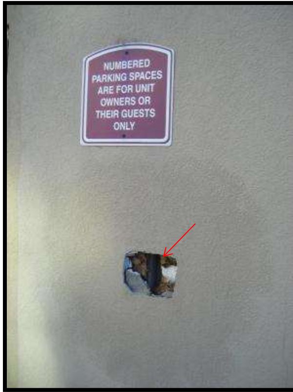
Photo 19: Hole in EIFS wall (North elevation).
