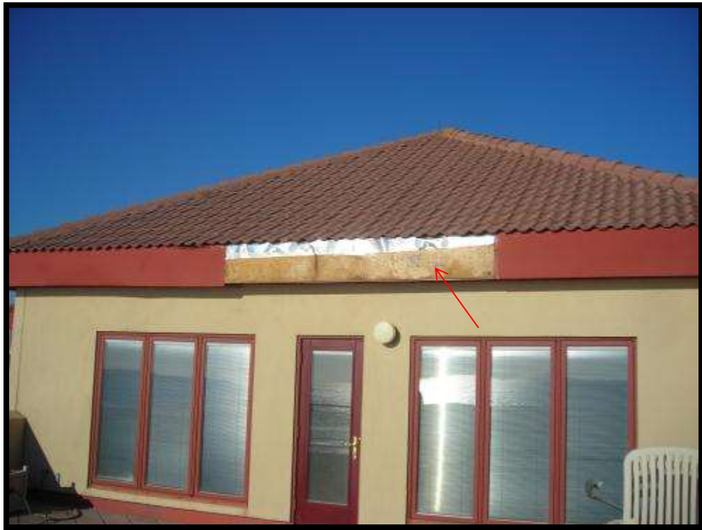
Photo No. 3: Damage to metal siding of upper roof fascia (View from balcony of Unit 701).
