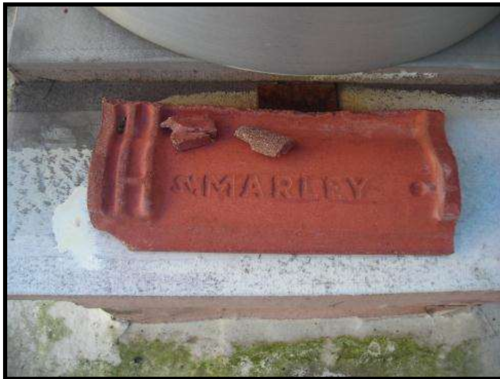
Photo 14: View of dislodged concrete roof tile.
