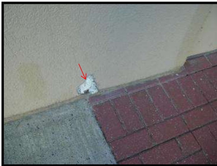
Photo 20: Gouge in EIFS wall (North elevation).
