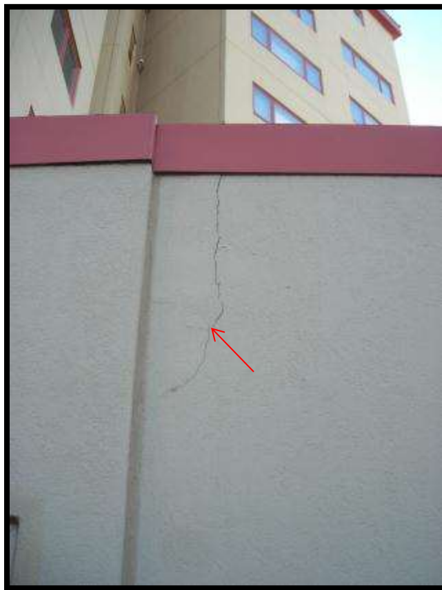
Photo 24: Hairline/minor crack in CMU block wall (North elevation).
