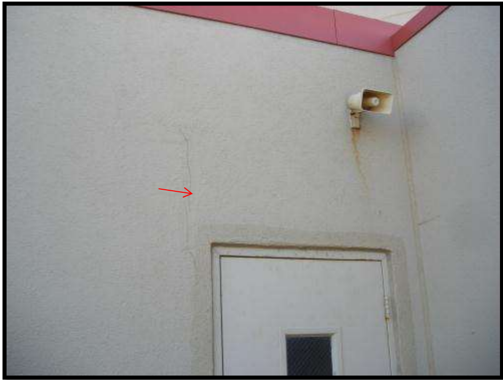
Photo 25: Crack in exterior first floor level wall (west elevation).
