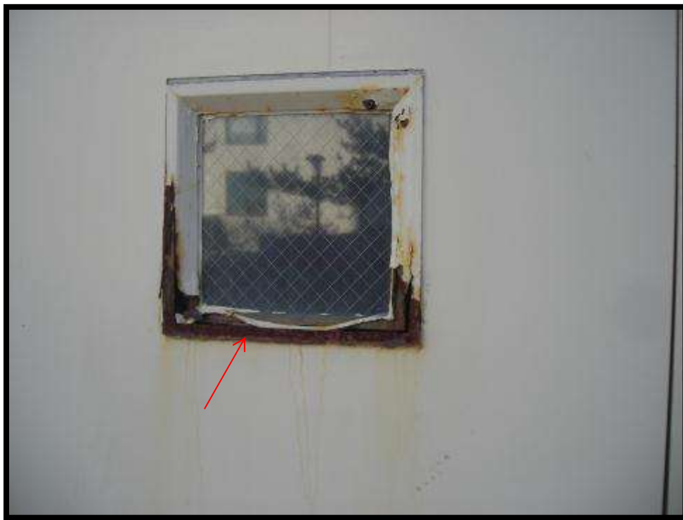
Photo 22: Damage to metal frame surrounding window of metal door (North elevation).
