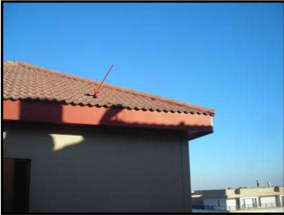
Photo 7: View of missing/dislodged roof tile (View from low-sloped upper roof).
