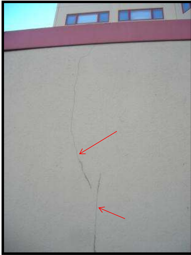
Photo 17: Hairline crack in CMU block wall (North elevation).
