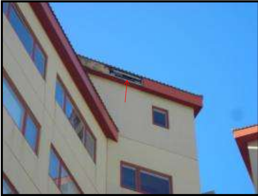
Photo No. 5: Damage to metal siding of upper roof (East elevation).
