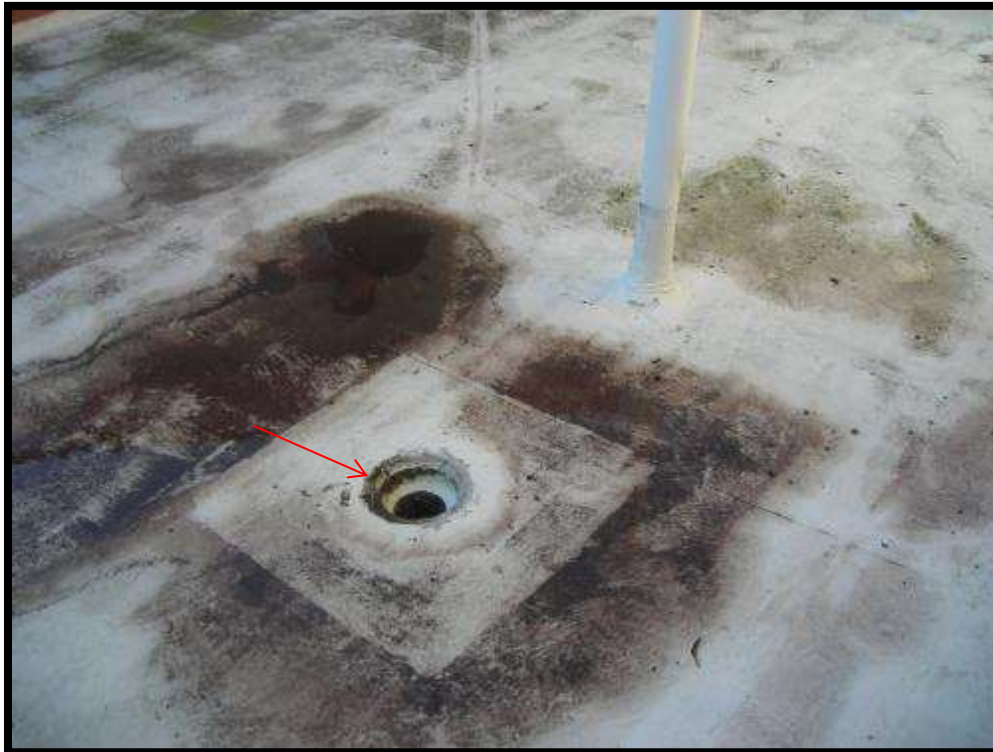
Photo 10: View of missing screen from field roof drain.
