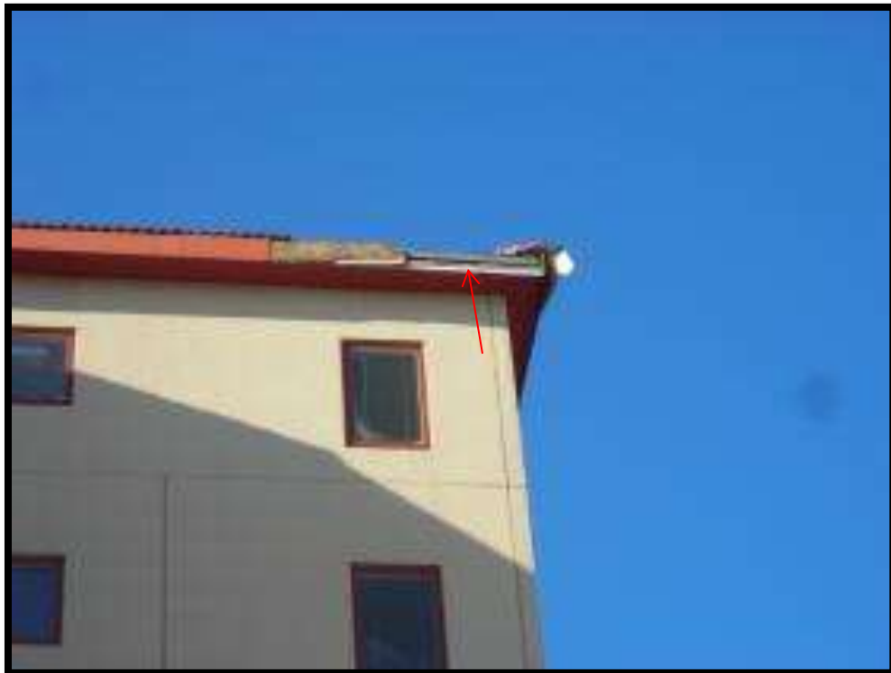
Photo No. 4: Damage to metal siding of upper roof fascia (North-east corner).
