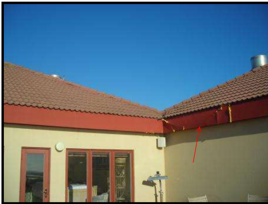
Photo No. 2: Damage to metal siding along upper roof fascia (View from balcony of Unit 704).
