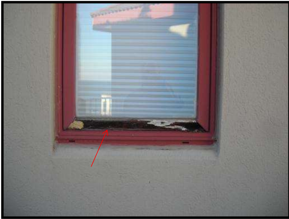
Photo 11: View of damage to bottom sash of window (Unit 704).
