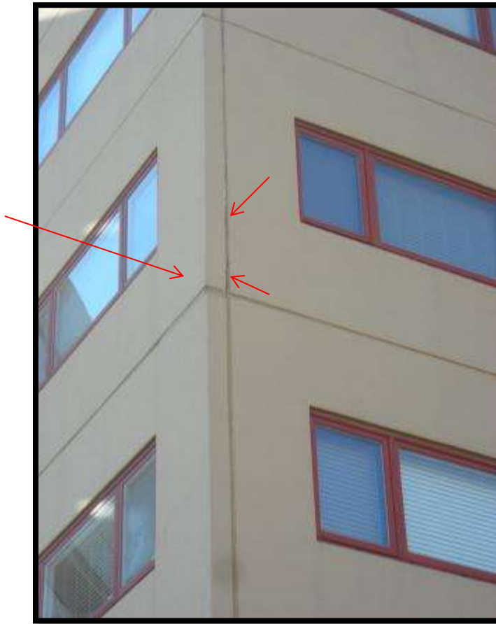
Photo 15: View of damage to EIFS wall panel along corner of building (North-east corner).
