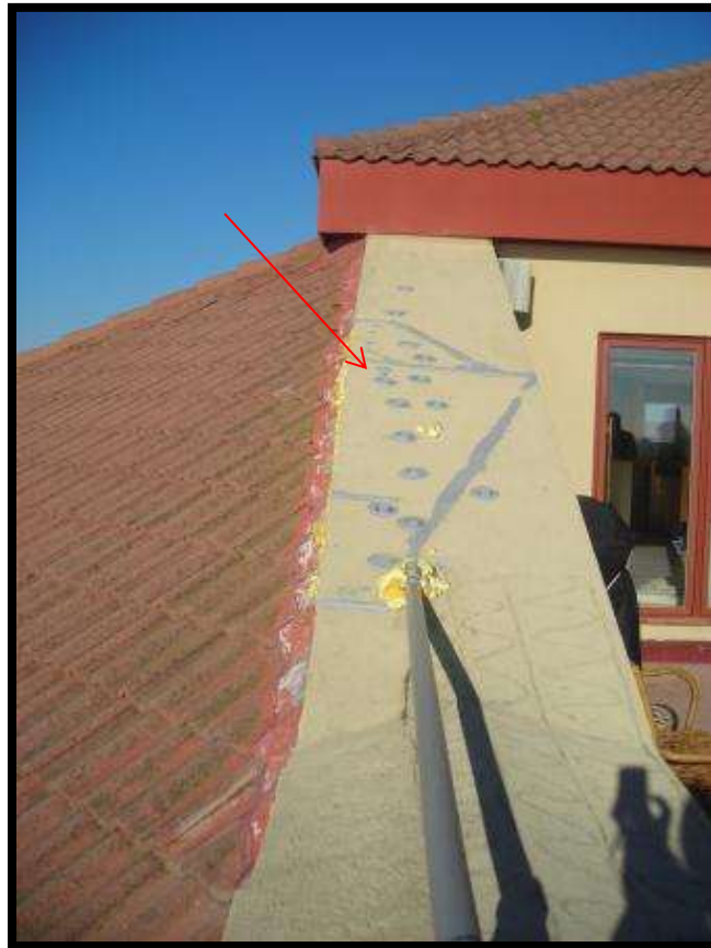
Photo 12: View of sloped EIFS wall cap damage (View from balcony of Unit 704).
